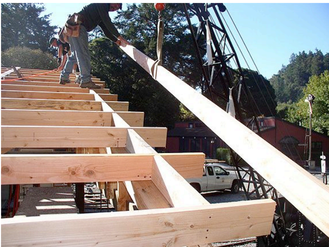
Fascia board ready to install on West end of car barn storage building.
