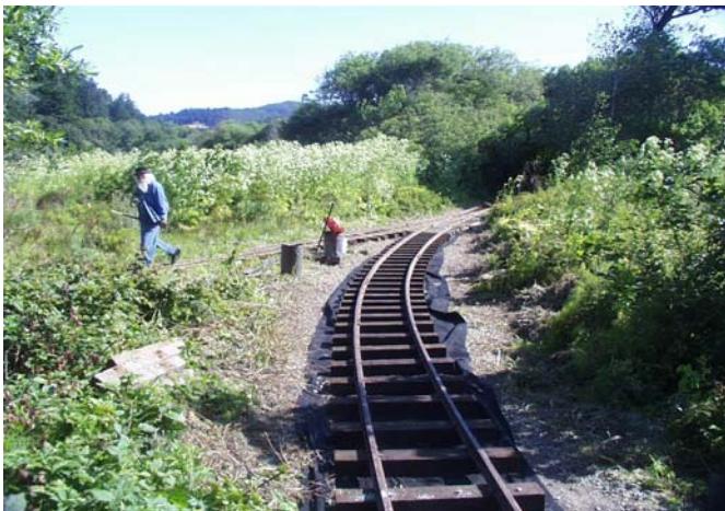
Photo 2 Title: Track before Ballast It shows Replacement of ties and Under lay-ment; the area is beginning to look a lot better.
