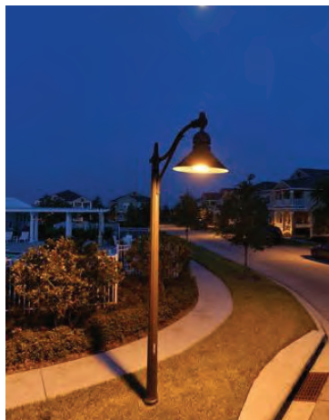
Figure 4.18 Example of Streetlight
