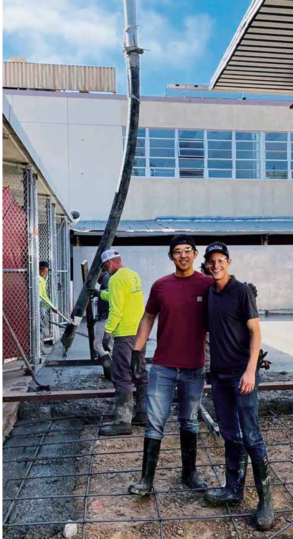
▲ Steven Zheng (foreground, left) and Nathan Horst renovated a concrete slab around the CAED's Support Shop. A CalPortland crew (background) was among the industry partners who donated materials and services.
